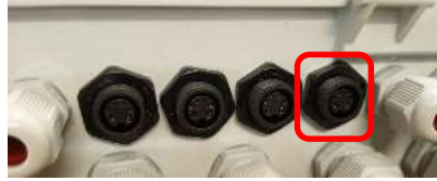
Figure 9 – Modbus Hub sockets on the CCU/DCCU
